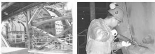
Figure 13. General view of one of the grinding mills that was treated by UP (left) and application of UP for rehabilitation of a weldment region in the grinding mill (right).
